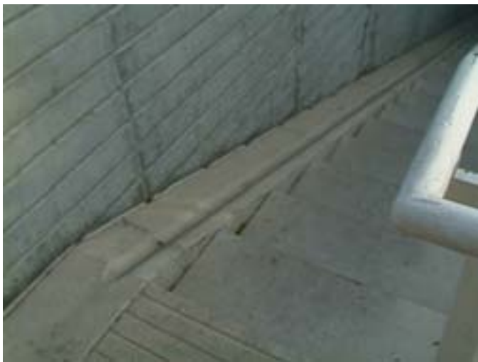
Channel for bicycle wheel in concrete staircase at McDonald's Cycle Centre, Chicago.
