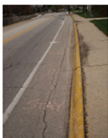
A bicycle lane with cracks, count as Few Impediments .
