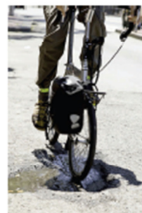
Street pavement with large holes, counts as Large Impediment .
